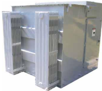
SUB STATION TRANSFORMER
